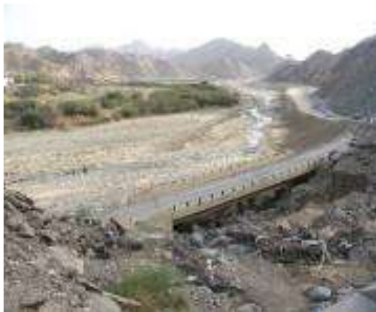
Damage of road structures by flood in South Western Saudi Arabia (ACSAD, 2008)
